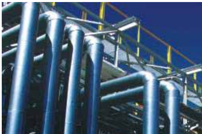
Photos: Details of installations at PCC Rokita S.A. - Brzeg Dolny near Wrocław, Lower Silesia
