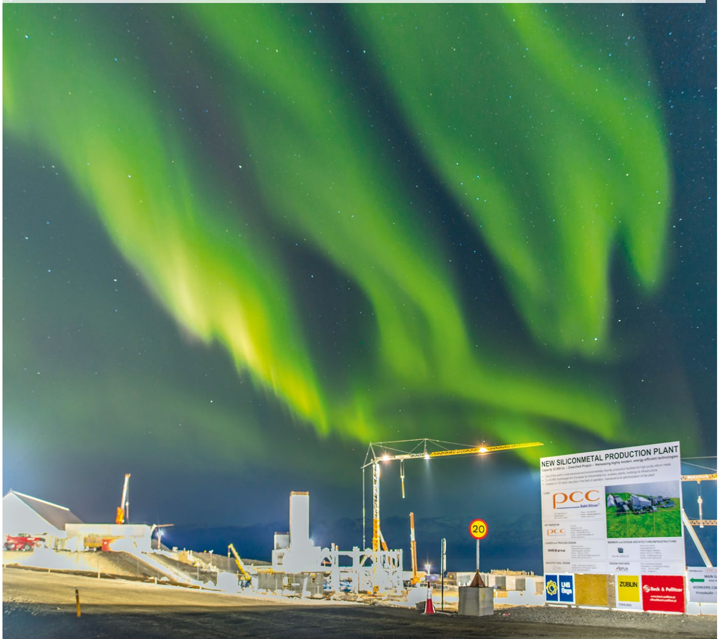
Northern Lights above our construction site near Húsavík in the north of Iceland. Here, PCC BakkiSilicon hf is in the process of constructing one of the most advanced and also most environmentally friendly silicon metal plants in the world, due for completion in 2018. On the left in the photo is the already finished coal storage facility (see also page 4).
