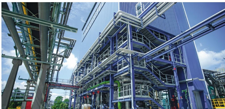
Due to high demand, all five production lines for polyether polyols of PCC Rokita SA at the Brzeg Dolny site are currently operating at full capacity. Measured in terms of standard polyols, total capacity currently stands at 110,000 metric tons per year.
